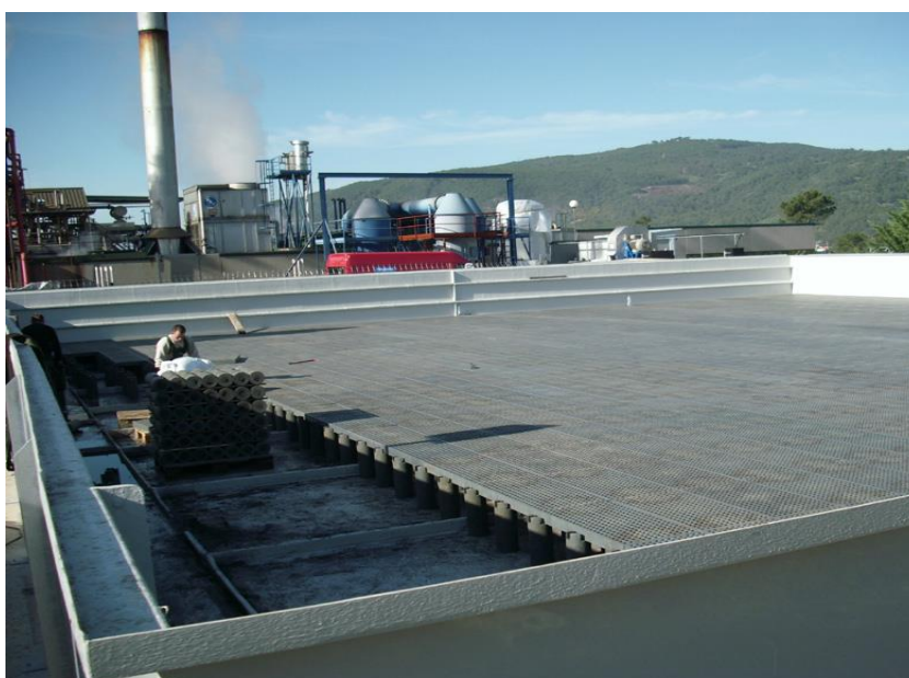
Figure 1-1 Hahn Plastics Ltd biofilter floor system at Montpellier, France.
